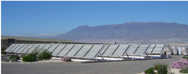
Fig. 13. View of the solar detoxification demonstration plant erected by ALBAIDA at La Mojonera (Almería, Spain), (Malato et al., 2007).
